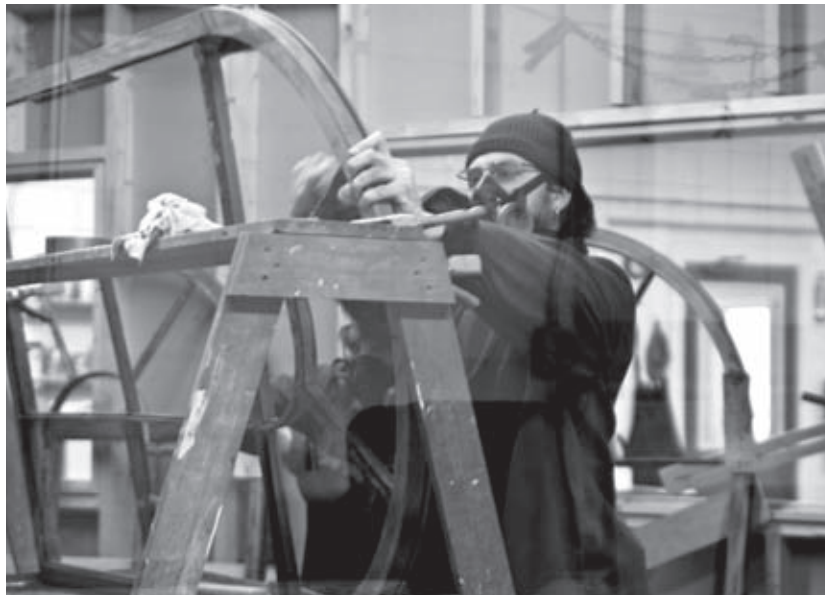
Restorer-builder Christopher Davis learns best practices of windows restoration: "Marc Bagala is a master at this craft."
